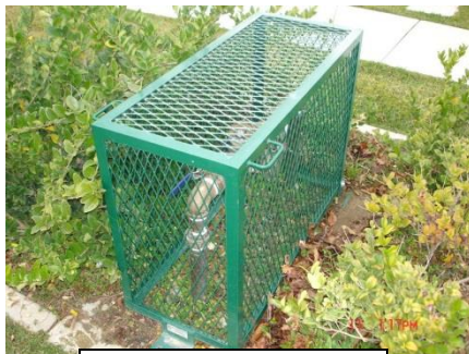
Backflow device with cage
